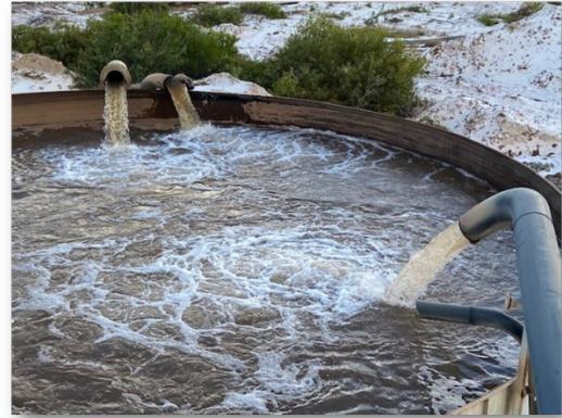
Optimised dosing at the thickener producing low turbidity overflow water
