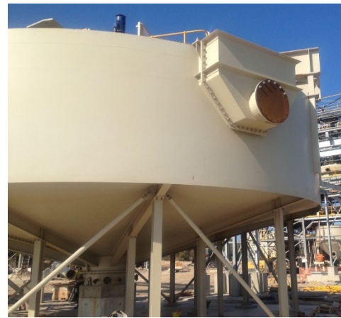
Thickener at the processing plant
