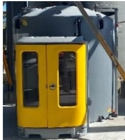
Self-contained chemical storage & dosing unit.
